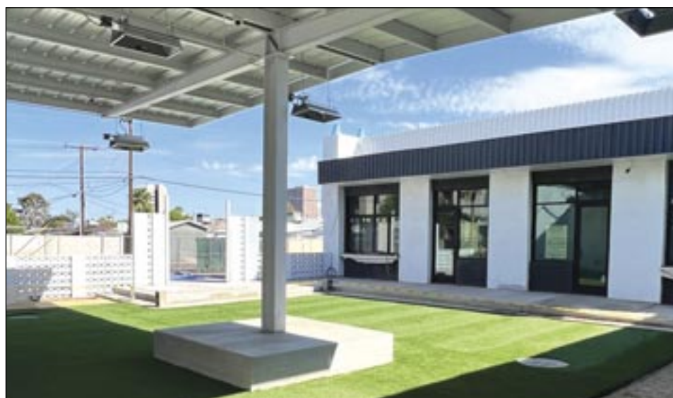
Construction is moving along on The Royale Commons, shown here facing southeast towards the main entrance off of 6th Drive, and towards retail spaces for Window Coffee Bar and STEMSWAG Floral & Gifting (submitted photo).
