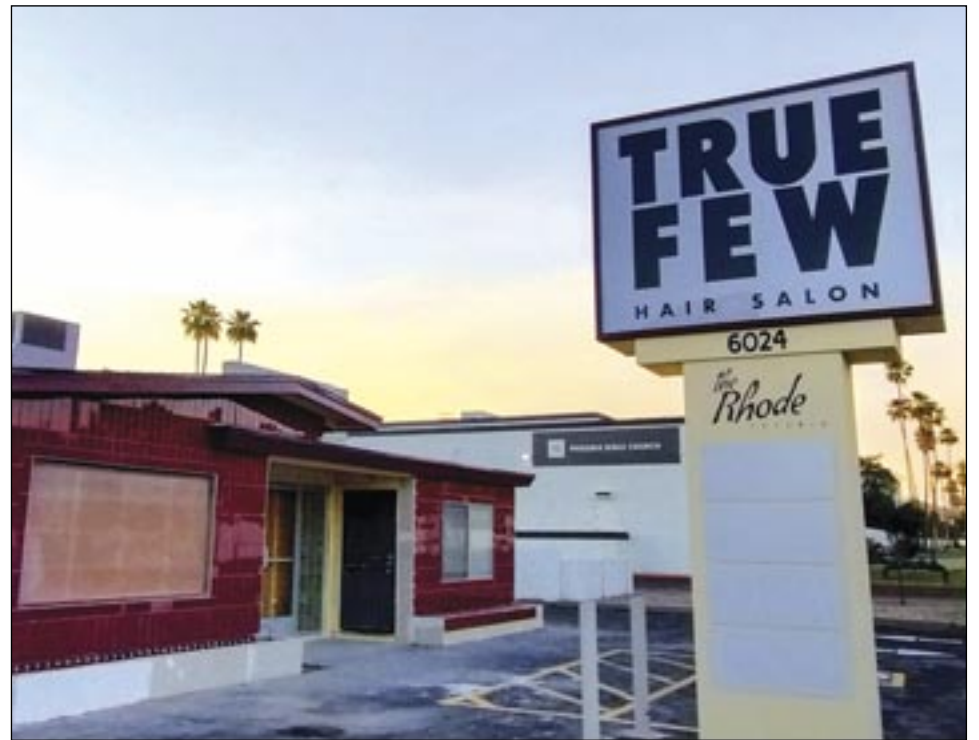
Work on the exterior of The Rhode, located at 6024 N. 7th Ave., was underway in April as True Few Hair Salon prepares for a May opening (photo by Kathryn M. Miller).
